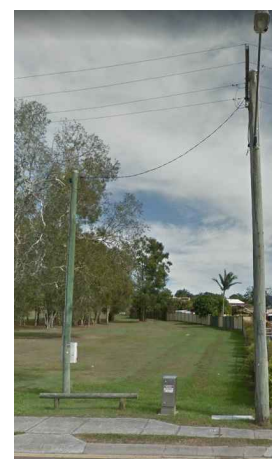
OVERHEAD SUPPLY FOR SWITCHBOARD
