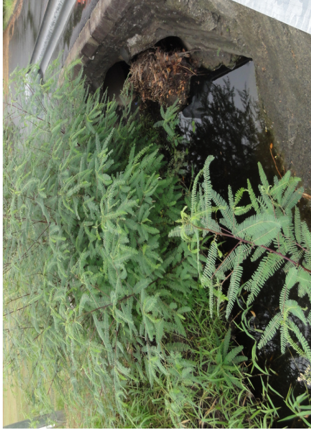
Photo 2 - Structure Detail (inlet blockage)
