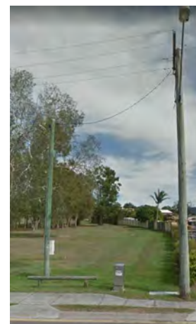
OVERHEAD SUPPLY FOR SWITCHBOARD
